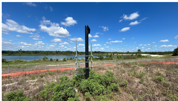
Above-grade vent at the nCino Sports Park
